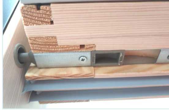
WINDOW BLOCKED - - the latch is extended
